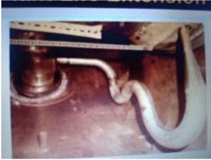
Top View of one of the critical piping – serpentine bends with envelop – Restricted Space – for Radiography before thermal insulation
